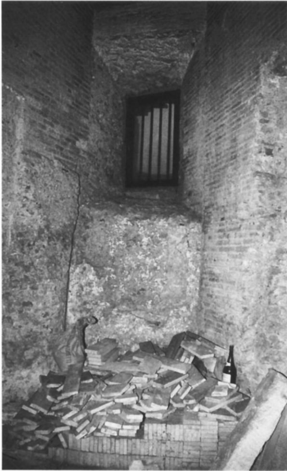
Fig. 18. View of construction joint in E.IV.12. Note that the left side of the window jamb is unfaced whereas the right side is faced showing that it existed before the wall to the left was added.
