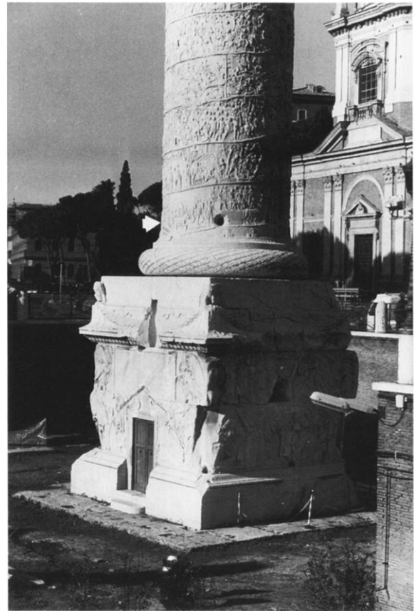
Fig. 10. Photo of lower portion of Trajan's Column. Travertine foundation cap is visible at base of pedestal. Arrow indicates the joint between two blocks with a robber hole where a connecting dowel has been removed.
