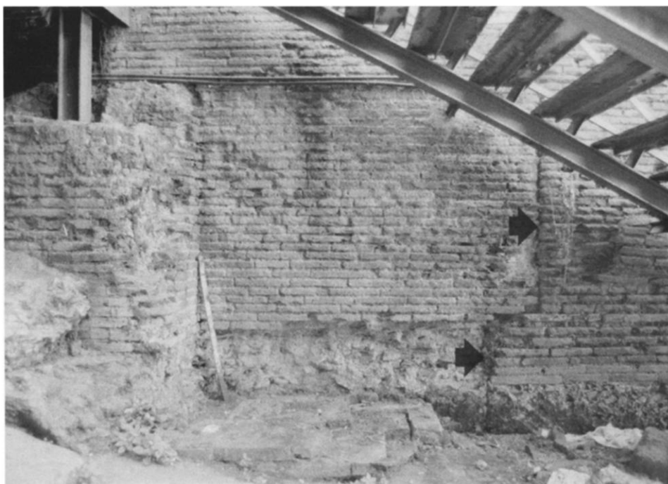
Fig. 23. Detail of west joint (W on fig. 22, indicated with arrows) on north facade of Aula
