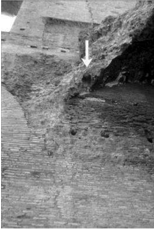
Figure 7. Porch, north end. Traces and remains of a terracotta tube, still well preserved, at the spring of a cross vault, placed perpendicularly to the exterior limit of the upper wall.
