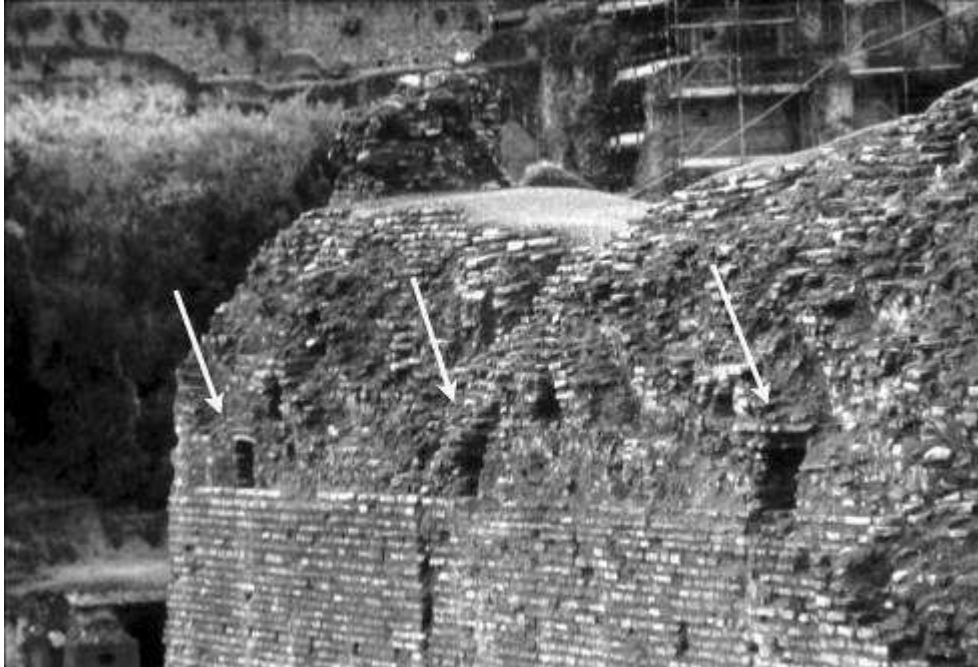
Figure 9. South-west perimeter wall, interior. Clearly visible the rectangular holes created along the springing line of the vault, marked by a course of bipedales , connected with the reference tubes. Each cavity is cm. 45 large, cm. 35 high, cm. 124 deep, with bipedales on top.
