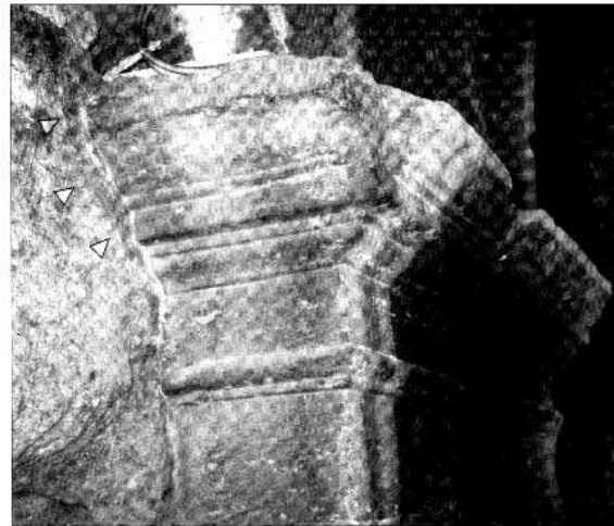
Fig. 26 Level I capital block on the travertine pier (position 3) at the end of wall 25/26. The arrows indicate where the tuff block of the wall has been cut away so that the travertine capital block could fit around it as shown in previous figure (right).
